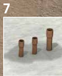
Leaking Penetrations i.e. Pipe Penetrations
