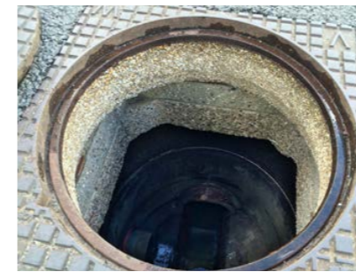
Manhole sewer entry after only 3 years in service exposed to biogenic corrosion.
