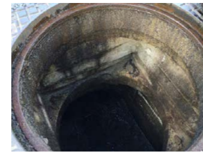
Manhole entry to storm water network after 3 years of service showing no deterioration.
