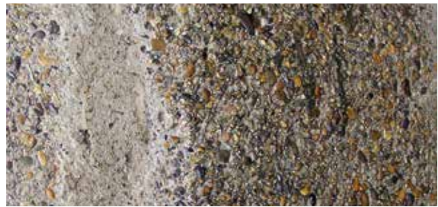
Due to continuous exposure, the cement film is eroded in an initial step, and thereafter larger and larger aggregates are rubbed, knocked or washed out of the hardened cement paste
