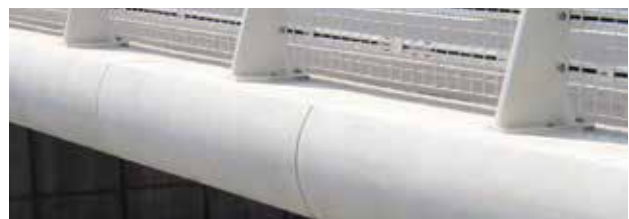
Highly stressed building components such as columns and beams are made of high strength concrete. High resistance to external influences also makes high strength concrete an ideal protective coating for exposed construction elements.
