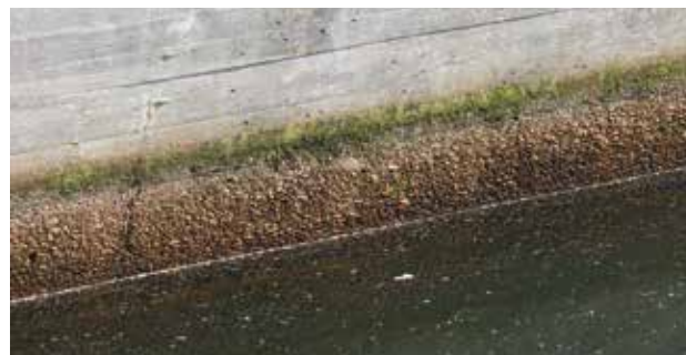
Heavy leaching and damage to the structural concrete are observed particularly in the water splash zone of biological treatment basins.
