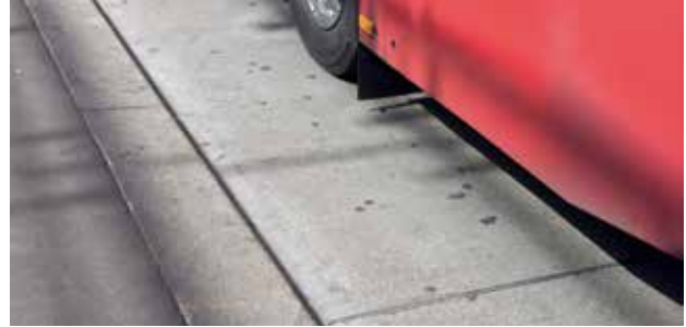
Concrete roadways and other publicly accessible areas, especially those experiencing high volumes of traffic or concentrated loads, are subject alongside high mechanical burdens also to strong abrasion, often presenting the risk of a smooth, slick surface.
