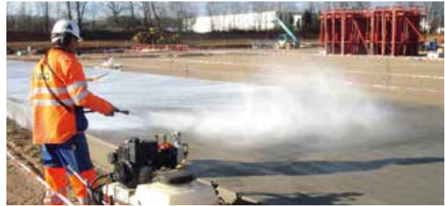
Immediate coverage or curing of concrete surfaces exposed to the elements is the most crucial step for protection of such surfaces.
