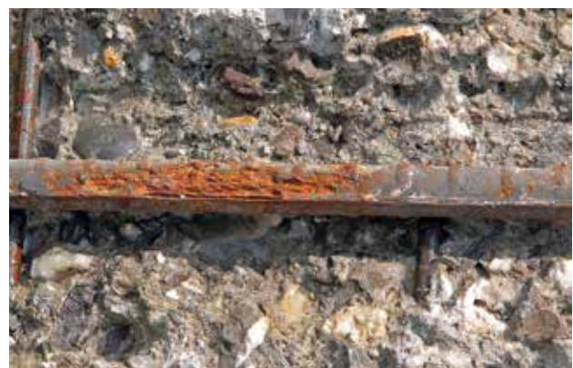
Damage to concrete structure due to insufficient concrete cover and low concrete quality
