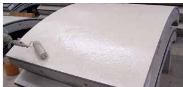
Immediately following curing in a steam channel, the concrete surface of tunnel lining segments is coated with water-based epoxy emulsion that is absorbed even into the smallest pores, thereby generating a sealed, protective coating.
