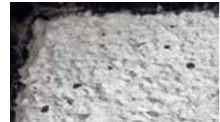
Very severe surface weathering
