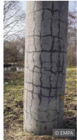
The appearance of ASR damage can be assessed very well on the drying concrete surface of this bridge pylon. Damage can appear within years or only after decades.
