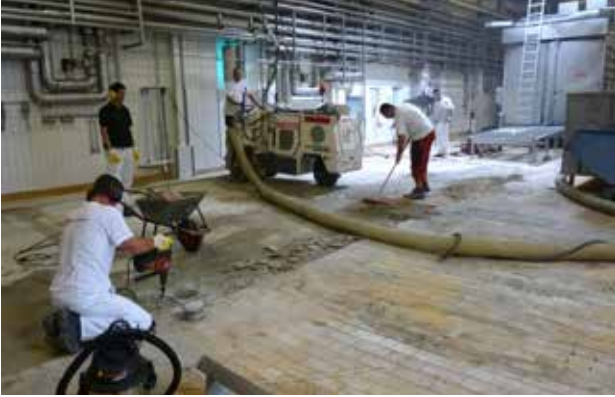
FRIDAY AFTERNOON: Mechanical removal of old tiles and epoxy adhesive. Substrate preparation and cleaning.
