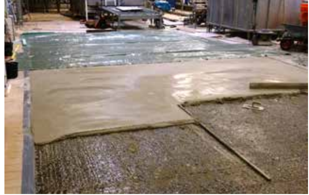
FRIDAY EVENING: Application of the bonding layer and the cementitious fast curing Sikafloor® HardTop-80 flooring screed.
