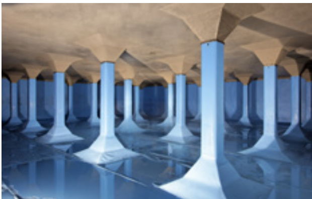
WATER RESERVOIR LUDWIGSBURG, GERMANY 2011
