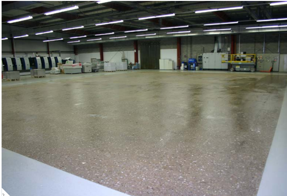
1 Strip installed concrete slab. 2 Floor grinded to tolerances in a free-movement area.
