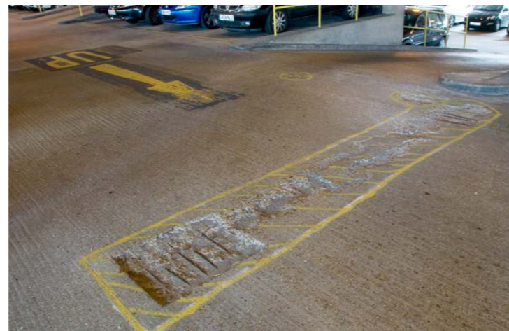
Aggressive chemicals degrade concrete. The picture shows damages of chloride attack from de-icing salts.
