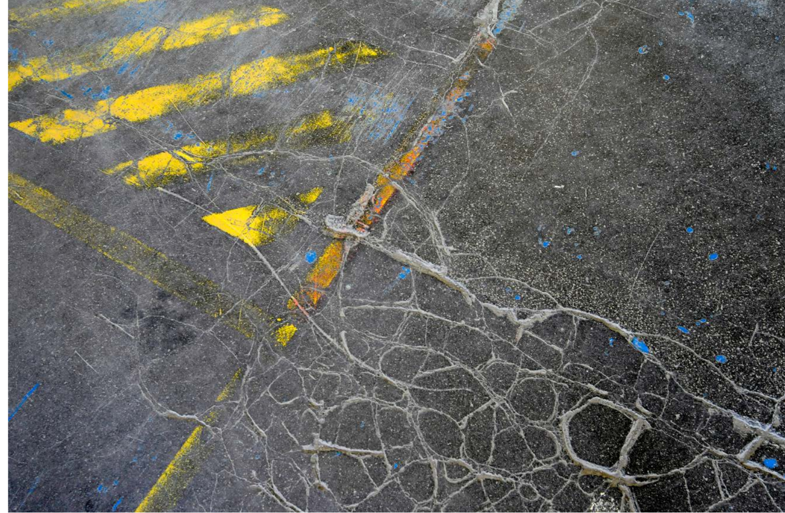
All cracks are not the same. Before repair remedies the cause of the cracks should be clarified.
