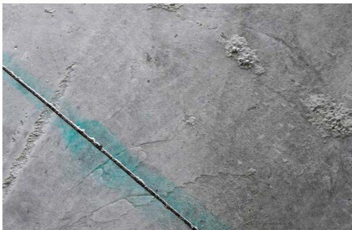
Surface defects due to bad finishing.
