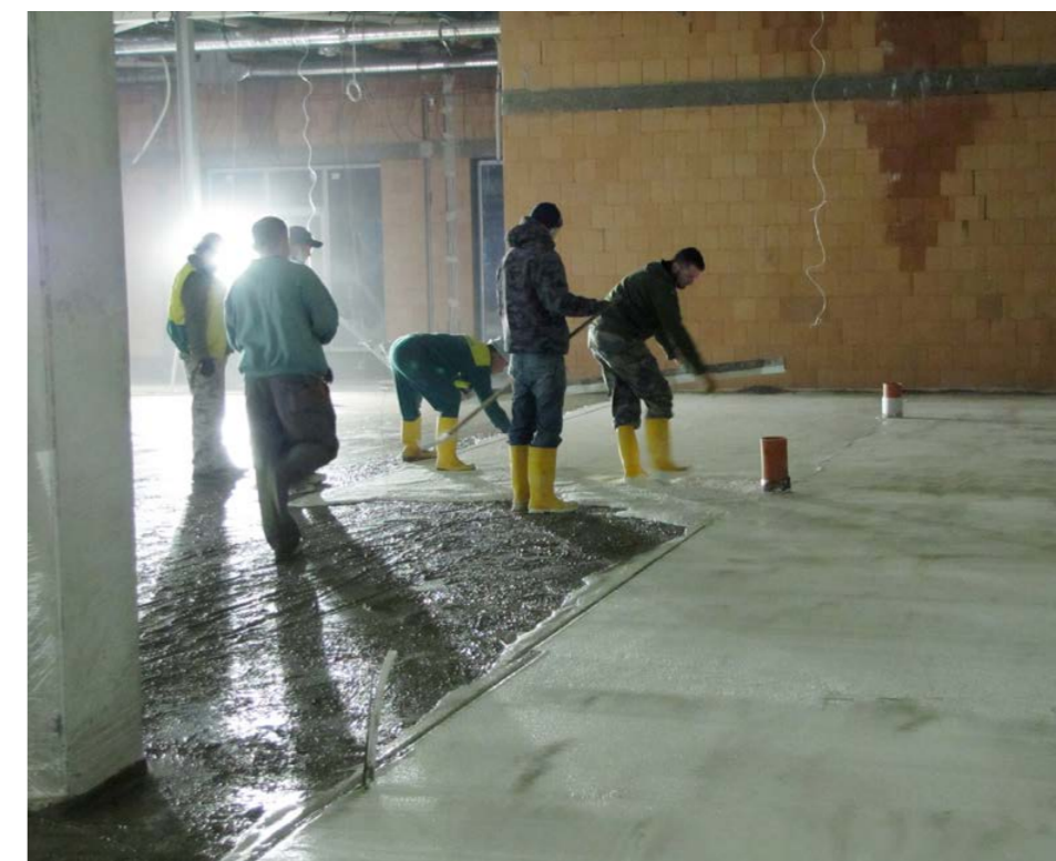
SikaFloor®-3+ CorCrete application in the building materials merchant Dek Znojmo outlet in Czech Republics. Refurbishment of 1200 m 2 concrete slab with the color Light Grey.
