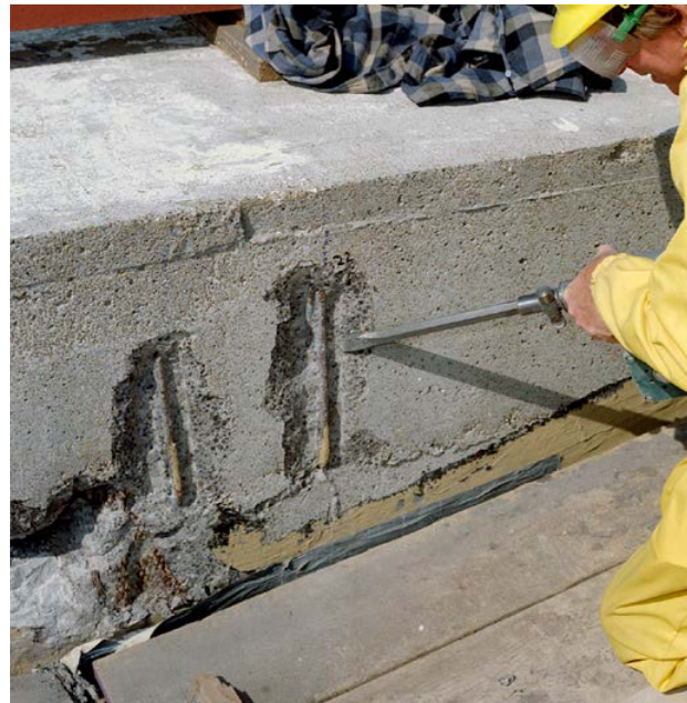
Damaged concrete structure
