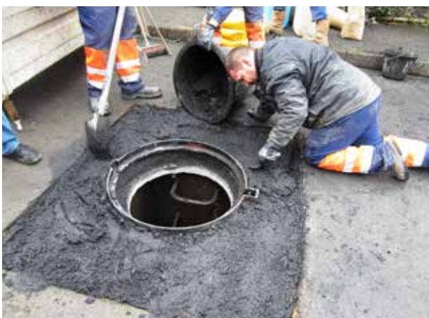
Pouring Sika® FastFix-138 TT to grout the manhole frame in position - mixed to a pourable consistency.
