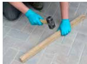
3. Compact well into the joints using a suitable Wacker-Plate, or simply use a wooden level and hammer.
