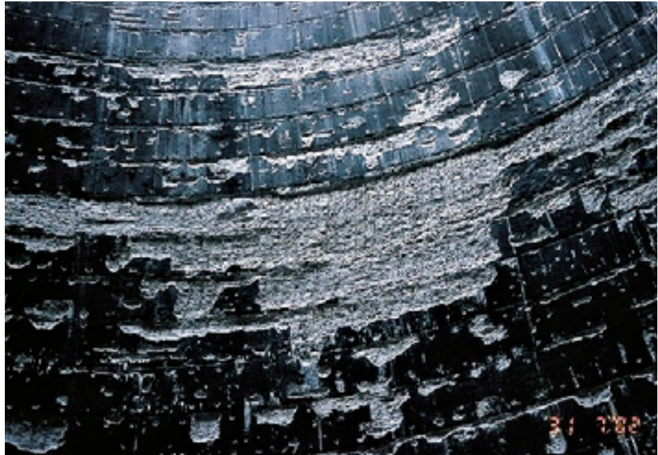
Severe corrosion of concrete and then of the steel reinforcement internally, despite a previously applied coating (coating was inadequate).
