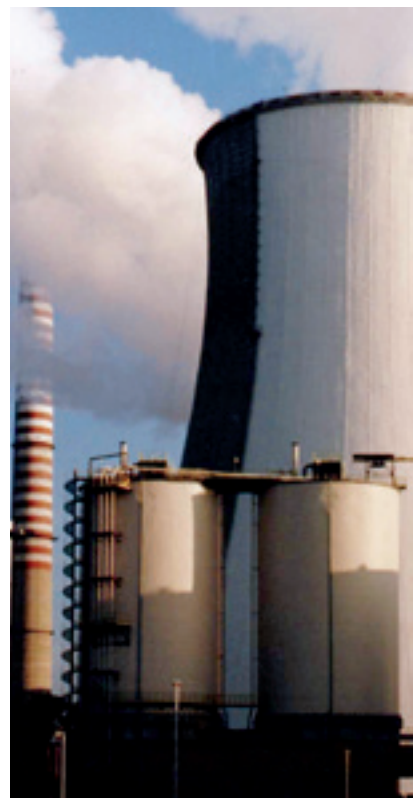
Sika protective coatings being applied to the external surfaces (all zones) of a cooling tower.
