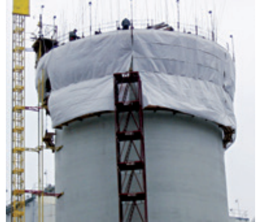
Right: Slip-forming a new concrete chimney base structure with Sika® ViscoCrete® technology.
