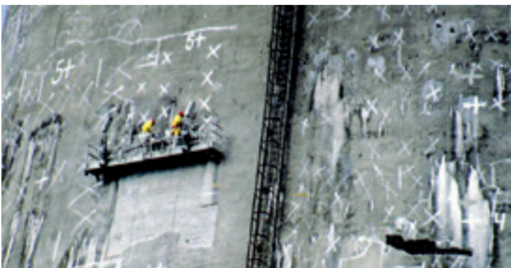
Break-out and removal of damaged concrete areas marked for repair in the condition survey.
