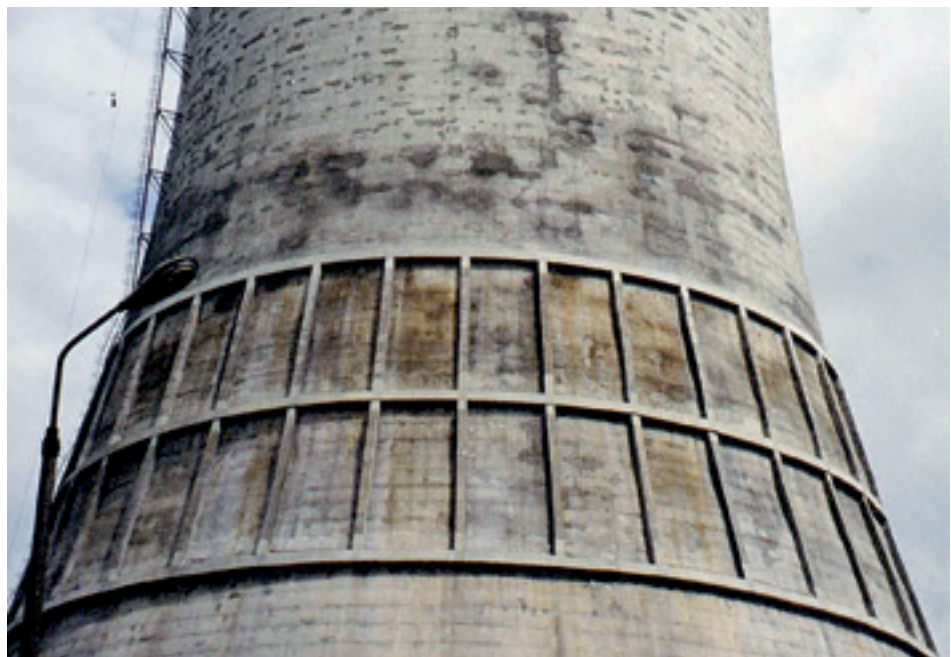
Carbonated concrete with spalling over corroded reinforcement accelerated by the steel being attacked by the acidic exhaust gases.
