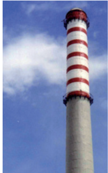
Aircraft warning colors using SikaCor® EG 5 as the top coating in zone 1 of a concrete chimney refurbishment.
