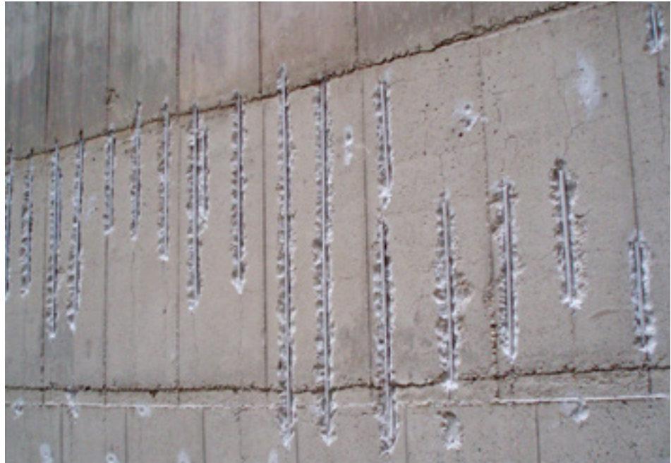
General corrosion induced by carbonation aggravated with low concrete cover issue.
