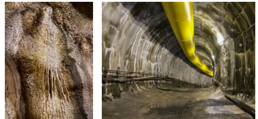
Fig 3.2: Damage due to insufficiently durable shotcrete (e.g. crystallization pressure due to sulphate attack)
