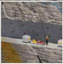
Stopping water inrush
