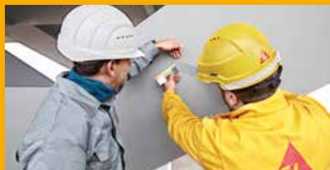
CORROSION AND FIRE PROTECTION
